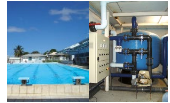
Guadeloupe, Basse-Terre Intercommunal pool Olympic sized 25x50m 5 filtres PP-2350
