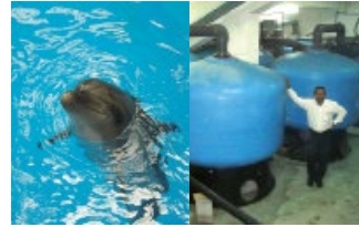
United Arab Emirates, Dubaï Dolphinarium, 3400 m 3 Intercommunal 6 PP-2000 filters
